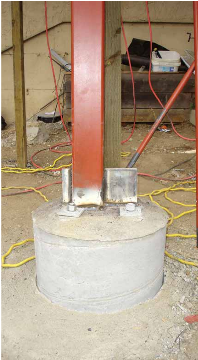
Figure 1. The multistory deck is anchored to the hillside by five 20-foot-deep reinforced concrete footings. Two of the footings support a steel moment frame, which is welded to 1-inch-thick steel plates fitted with 24-inch-long anchor bolts embedded in the concrete.
