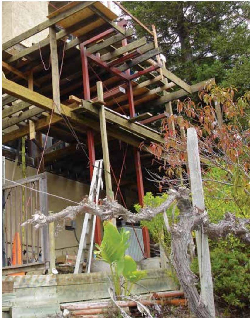
Figure 2. A three-story steel moment frame reinforces the deck framing against lateral loads, and helps support some of the framing. The frame was welded together on site from 6-inch by 6-inch steel columns and 6-inch by 8-inch steel cross members.
