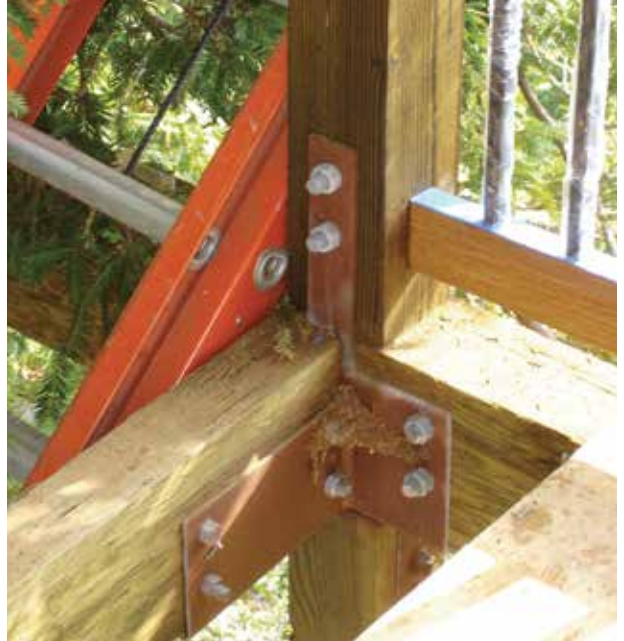
Figure 6. Custom-fabricated brackets attach the wood framing to the steel moment frame where required.
