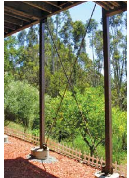
Figure 3. The moment frame is diagonally braced with 1-inch-diameter threaded rod, which is bolted to brackets welded to the steel columns.
